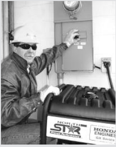
Great Lakes Energy's Dave Matz points out the safety transfer switch that allows this portable generator to be safely connected to the home.
